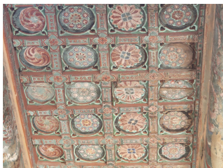
Fig. 42. Ceiling of the Daeungjŏn Hall in Pulguksa Temple (photo by author, May 24th, 2022).
